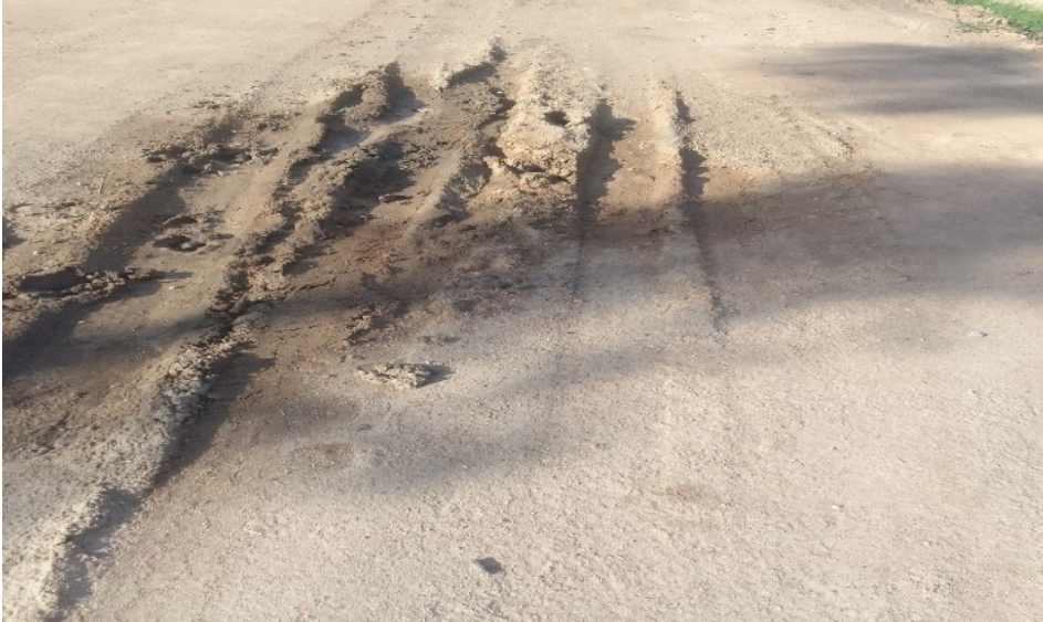
Figure 7: Road defects at Magulukende -Sukumas
