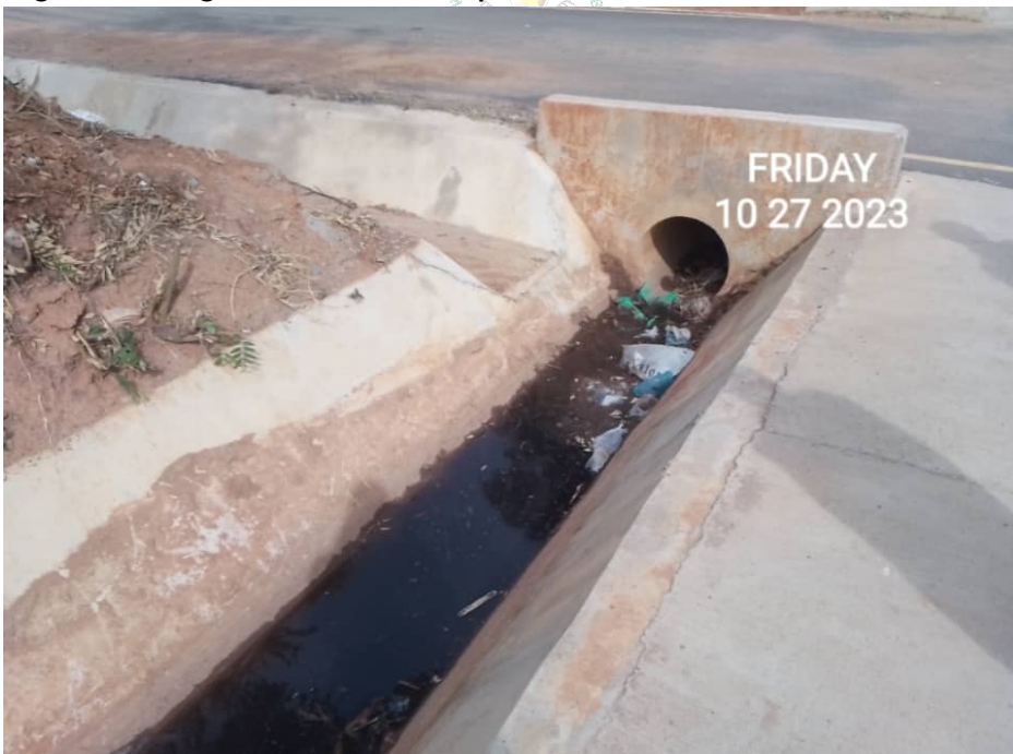
Figure 10: Stagnant water in the open drain
