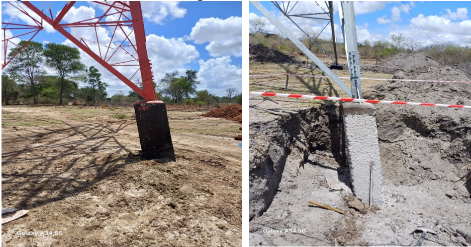
Figure 5: Inadequate backfilling around the tower's foundations.
