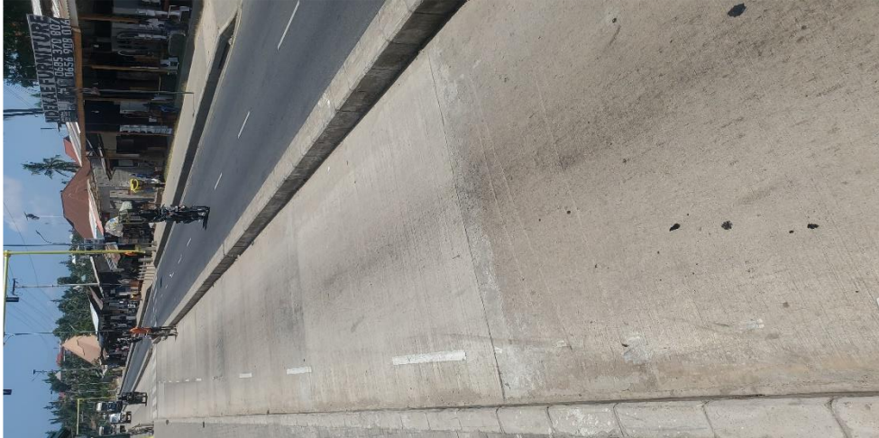
Photo 11. 2: Status of the Rectified rigid pavement sections at Mbagala-Kizuiani between 6+480 - 8+910 LHS. The Photos were taken by Auditors on 29 November 2024
