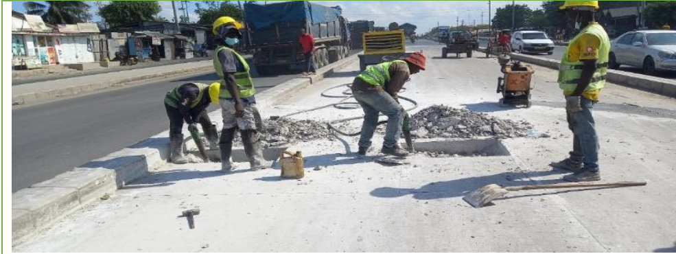
Photo 11.1: Contractor removing the defective rigid pavement sections as preparation for reconstructing them as they appear at Mbagala - Kizuiani between 6+480 - 8+910 LHS. The Photos were taken by Auditors on 17 November 2022.
