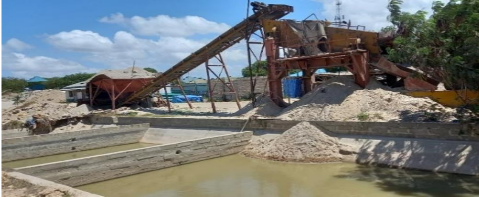
Photo 11. 3: Special equipment to wash/clean sand from deleterious materials for BRT Phase 2. The Photo taken by Auditors at Mbagala Contractor’s Campsite on 16 November 2022
