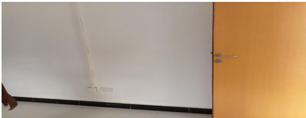
Photo 9.1: The ICT port near the entrance door at Mkuranga District Hospital.
