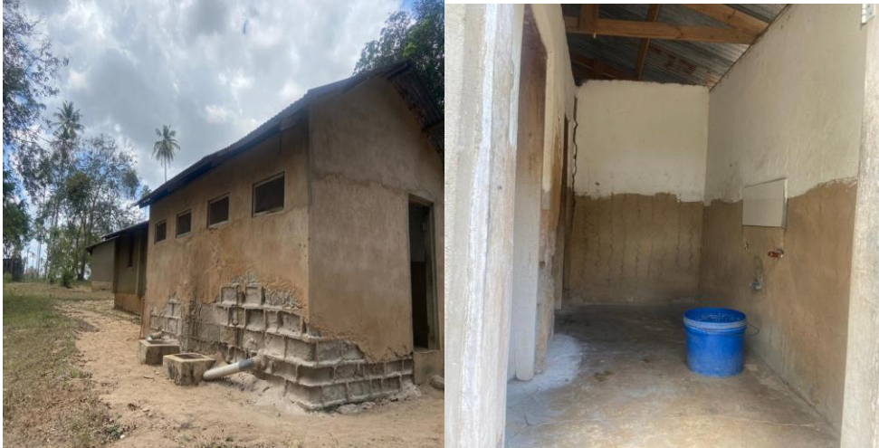
Photo 3. 4: Facilities (Washrooms) of Vikuruti rehabilitation village showing the washroom condition that needs to be renovated with no supply of water. This picture was taken by the Auditor on 26/09/2023.
