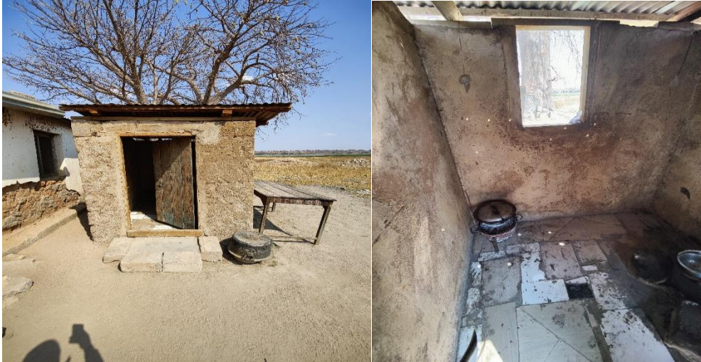
Photo 3. 6: Facilities (Kitchen area) of Hombolo rehabilitation village that need to be demolished and rebuilt. Photos were taken by the Auditors on 15/09/2023.
