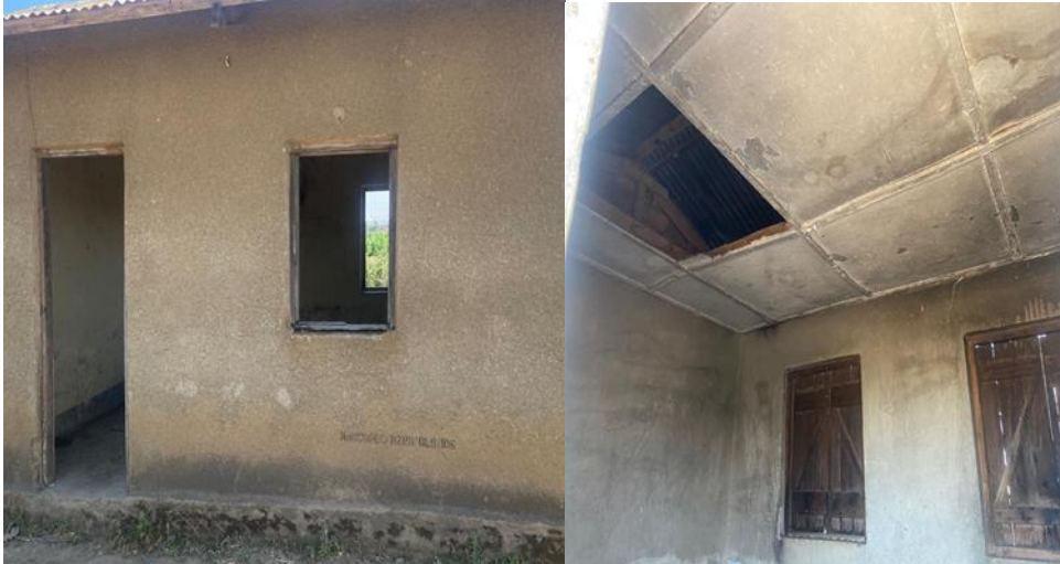
Photo 3. 4: Abandon facilities of Mbeya zonal rehabilitation village show building that needs to be renovated to function; picture taken by Auditor on 04/10/2023.
