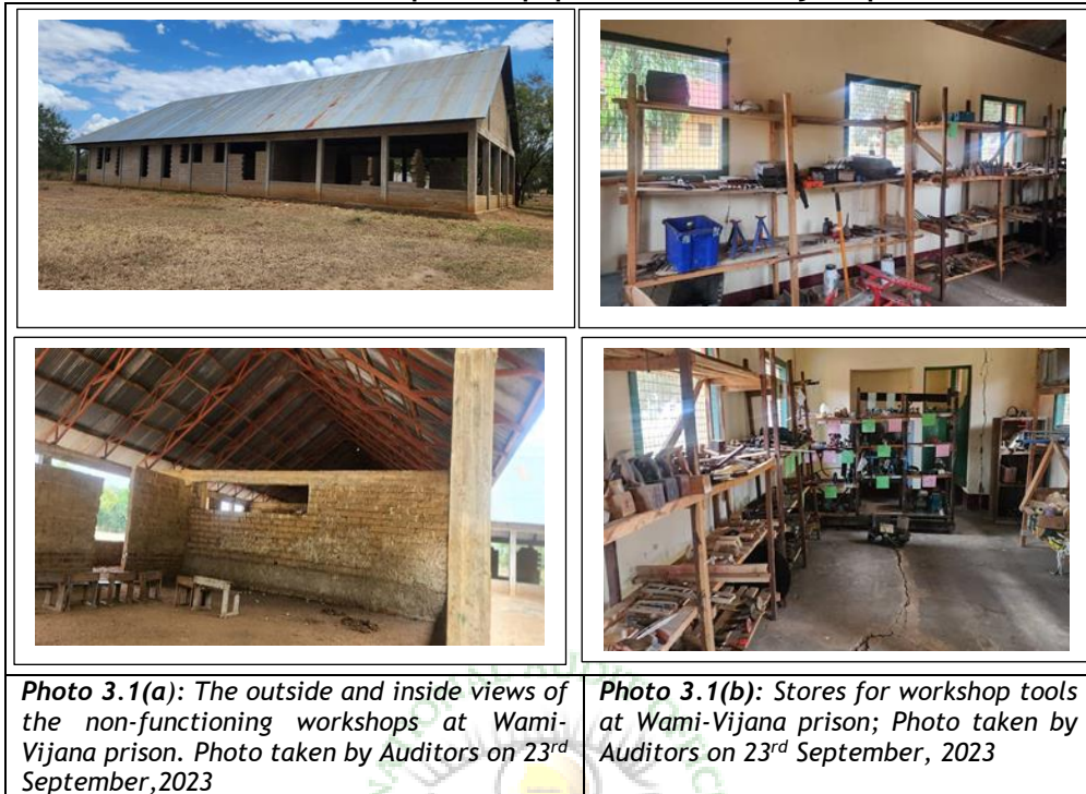
Photo 3.1: Workshop and equipment at Wami-Vijana prison
