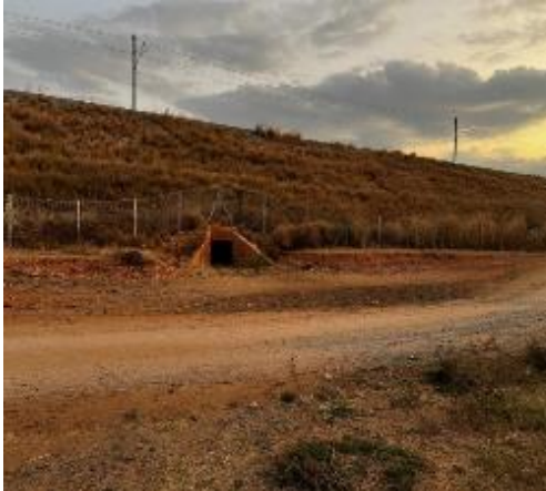
Photos 3.3(e): Box culvert under the Standard Gauge Railway (SGR) ridge for discharging stormwater from one side to another along the Standard Gauge Railway (SGR) ridge in Kilosa district. (Caption by Auditors in September 2024)
