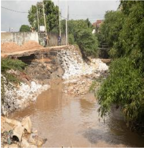
Photos 3.3(a): Banks erosion of the Tenge River due to the high speed of stormwater runoffs at Kigogo Ward in Kinondoni Municipality. (Caption by Auditors in July 2024)
