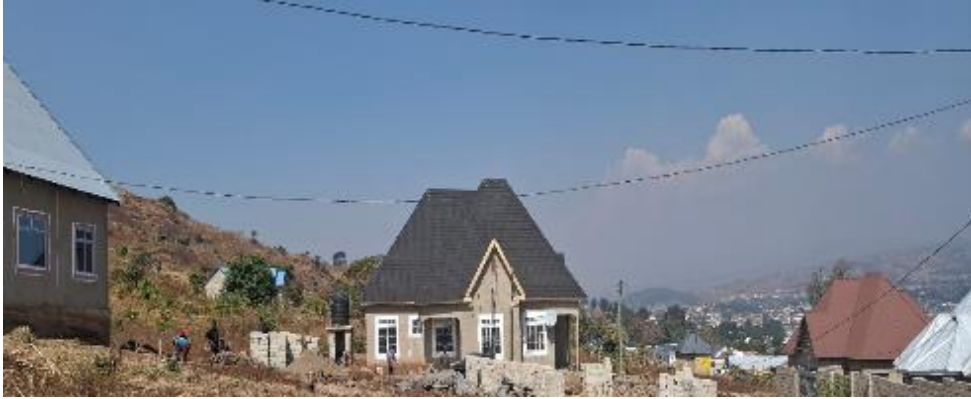
Photo 3.6 (c): Ongoing Construction at the Bottom of the Hill in Mbeya City Council (caption by auditors on 18 September 2024)
