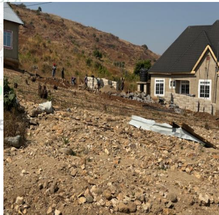
Photo 3.5(b): showing ongoing construction works in the flood-prone area by the Itezi dwellers in Mbeya Region (Caption by Auditors in September 2024)
