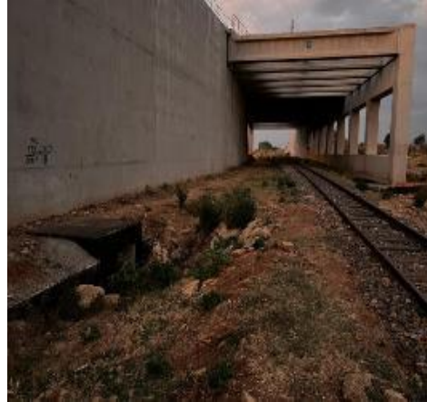
Photos 3.3(f): The other side of the box culvert where there is no continuation of the flood water discharge channel under the Mitre Gauge Railway (MGR) ridge, resulting in accumulation of flood waters affecting the neighbouring areas along the Standard Gauge Railway (SGR) ridge in Kilosa District (Caption by Auditors in September 2024)
