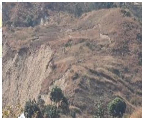
Photo 3.6 (b): Cracked remaining portion of the landslide as a hazardous portion (photo caption by auditors 18 Sept 2024)
