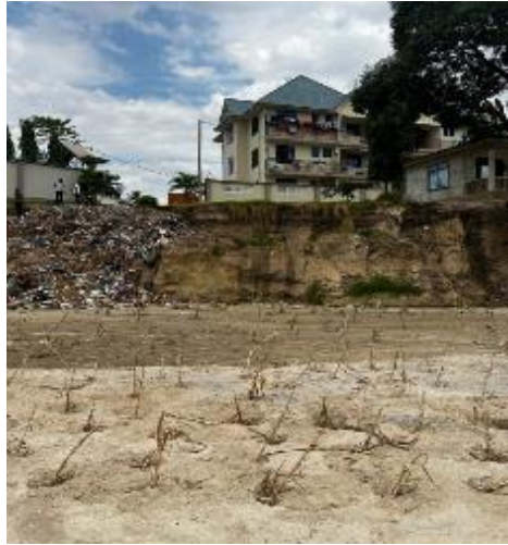
Photos 3.3(b): River bank erosion exposing the residential building to the risk of collapsing along the Nyakasangwe river at Boko ward in Kinondoni Municipality. (Caption by Auditors in July 2024)
