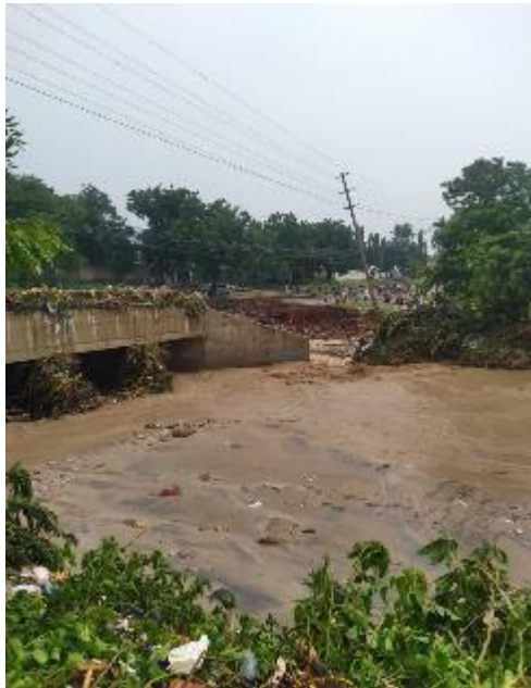
Photo 3.2(a): Stormwater carrying solid wastes leading to blockage of the waterway under the bridge caused by illegal dumping of solid wastes along the river banks.
