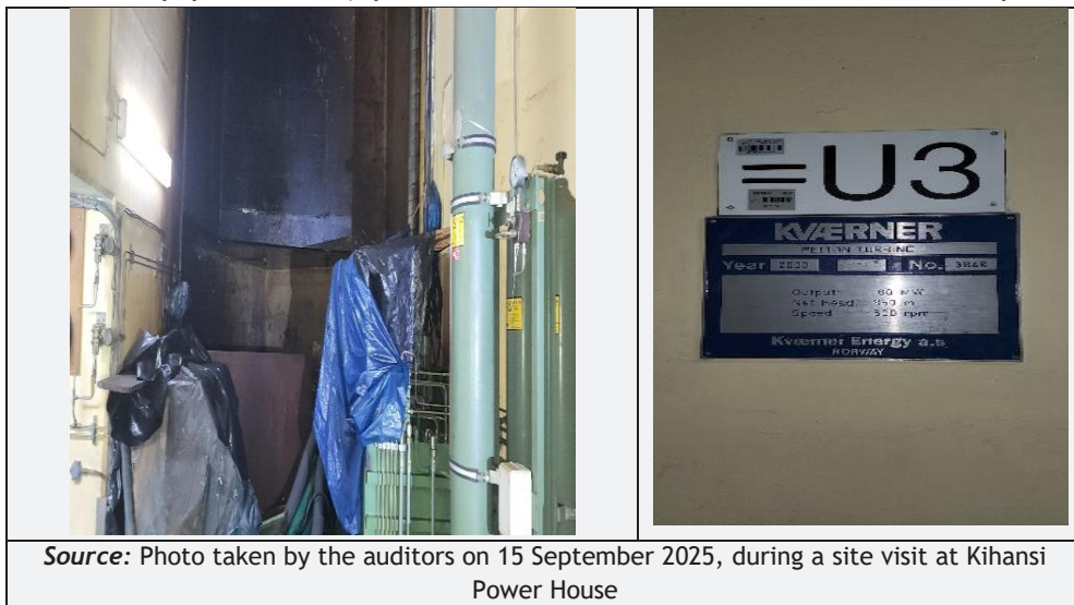
Photo 3.3: Turbine No. 3 is out of service at Kihansi Power House.
