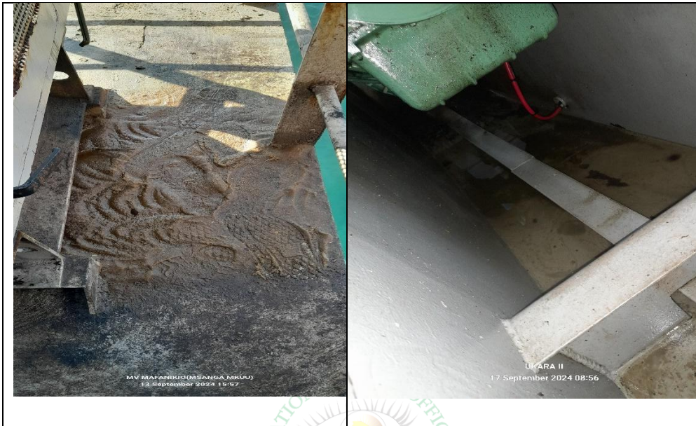
Photo 3. 1: Leakage of the Oil on the Engines
