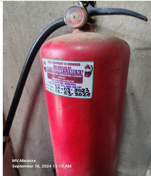
Photo 3.5(b): Expired Portable fire extinguisher as observed in MV Mwanza
