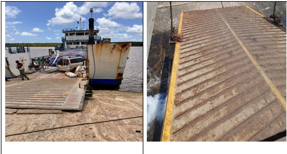
Photo 3. 2: Corrosion on the Hull Structure and Ramps
