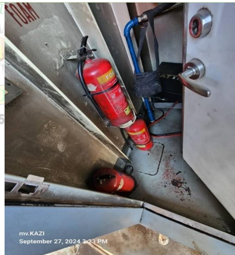
Photo3.5(d): Portable fire extinguisher placed in an inappropriate location at MV Kazi
