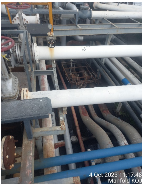
Photo 1: Shows the corrosion status of the pipelines at KOJ Manifold as of 4 th October, 2023
