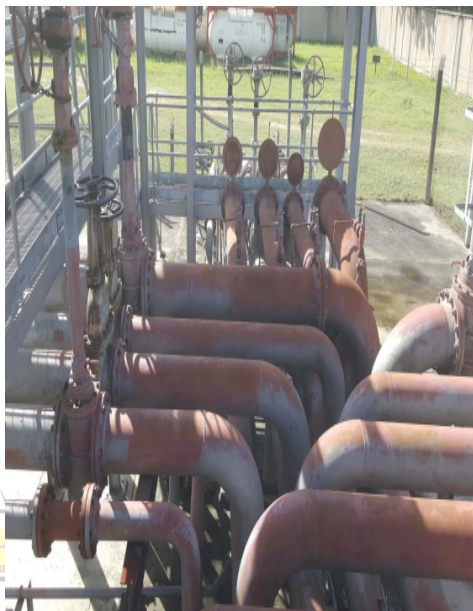
Photo 2: Shows corrosion status of the Diesel pipeline from KOJ to PUMA/GAPCO manifold 2
