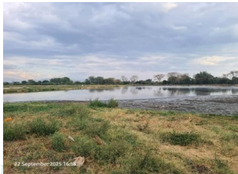
Photo 3.2: Waste Stabilisation Pond at Mabogini in Moshi, which has reached maximum capacity
