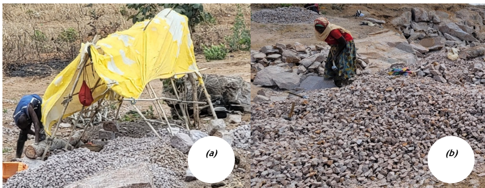
Photos 3.2 (a and b): Size Reduction of Aggregates using Low Mechanised Mining Equipment (Photos Taken by the Auditors During Site Visit at Chemichemi Quarry in Ruvuma Region on 22 nd September 2023)
